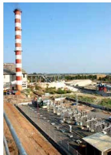
Switchyard at the cogeneration plant
