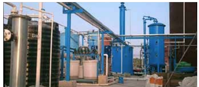
Condensate Polishing Unit (CPU): Capacity - 65 m/Hr. CPUs established in the sugar and distillery plant to collect the condensate water, treat it, and re-use it in the plant. Due to this the raw water consumption has been drastically reduced. Also the excess wastage water going outside the factory has been reduced.
