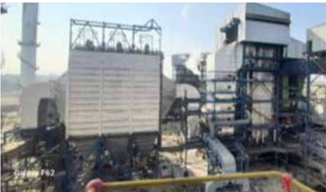
70% pith-fired boiler supplied at M/s Bindal Paper Mills Ltd. (Sugar Division) Bijnor by Isgec in year 2023
